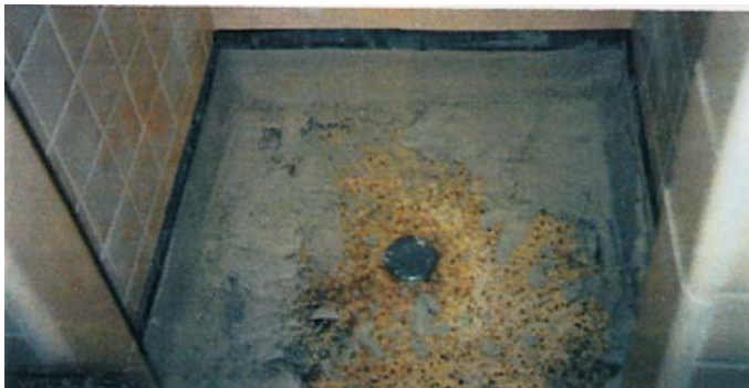
Leaking existing terrazzo shower pan. Note tape applied above the first course of tiles to neatly define the DuraQuartz repair.
