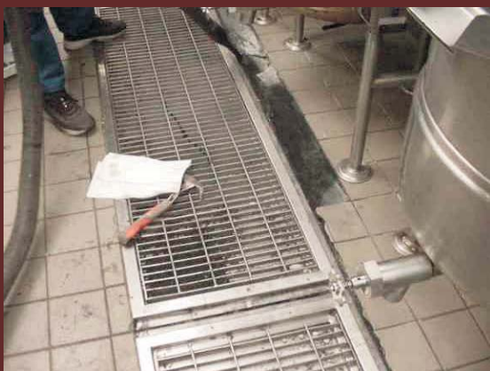
Some tiles were in such poor shape that they were completely removed.
