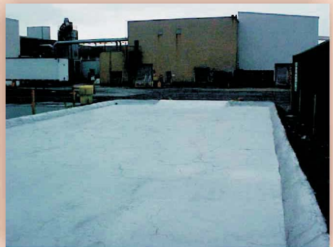
View from the opposite direction. Pallets containing drums of chemicals are stored here.
