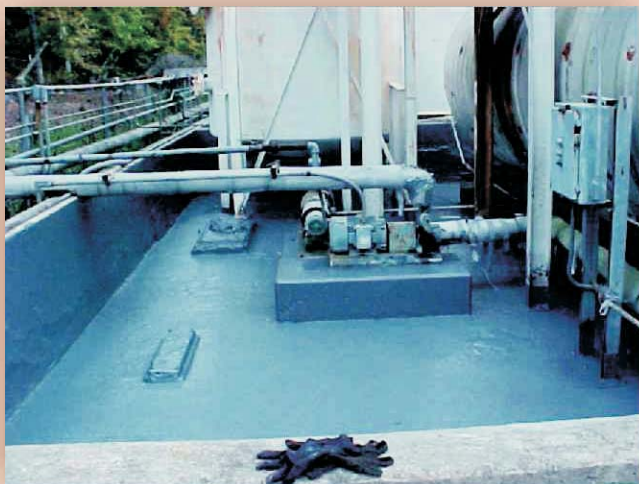
The second containment area was first power washed, cracks were repaired with DuraQuartz, P4C was applied over the concrete followed by 2 coats of CHEMCLAD SC.
