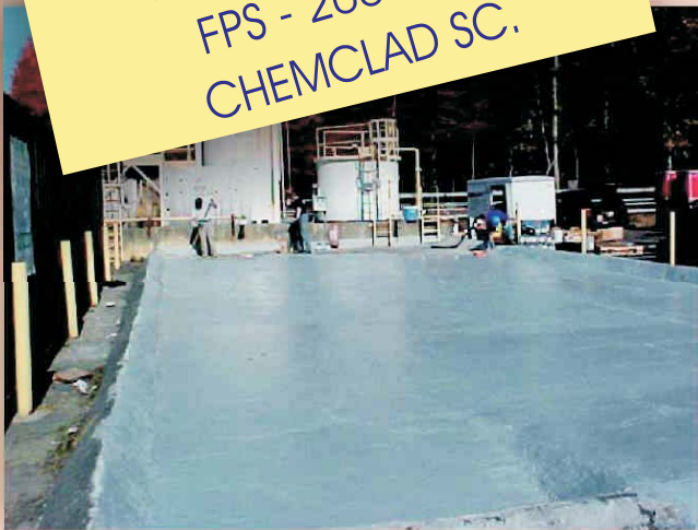
This, the largest of the three areas was first power washed, then abraded with a floor sander; cracks were repaired with ENECRETE DuraQuartz and then coated with ENECLAD FPS 2000.
