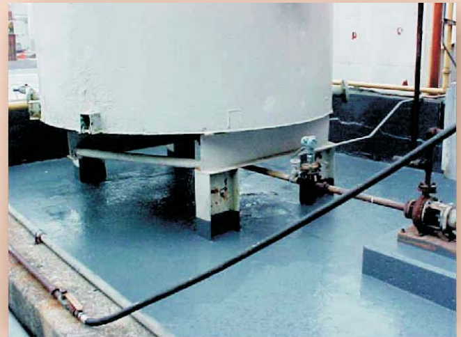
The third containment area was repaired and protected as per the second containment area.
