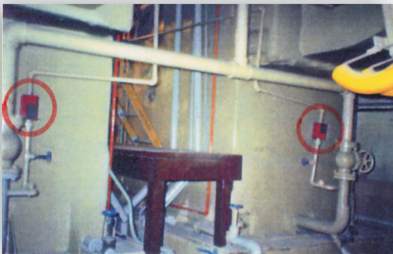
ENEFLOW 1000's installed on boiler make-up water lines.
