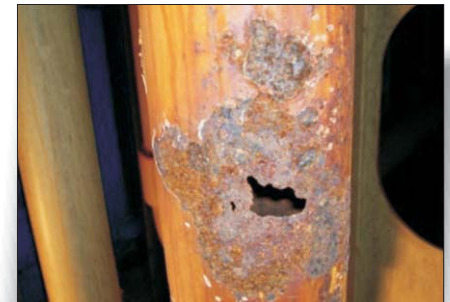
Holes caused by corrosion
