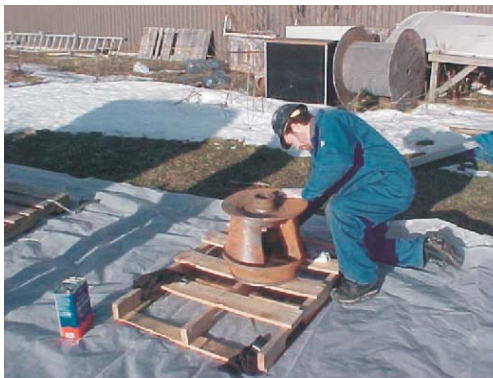
Impellers placed on pallets outdoors and then grit blasted to minimum 3 mil profile.
