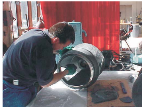
CeramAlloy CP + AC was used to smooth out and rebuild eroded areas of both impellers.
