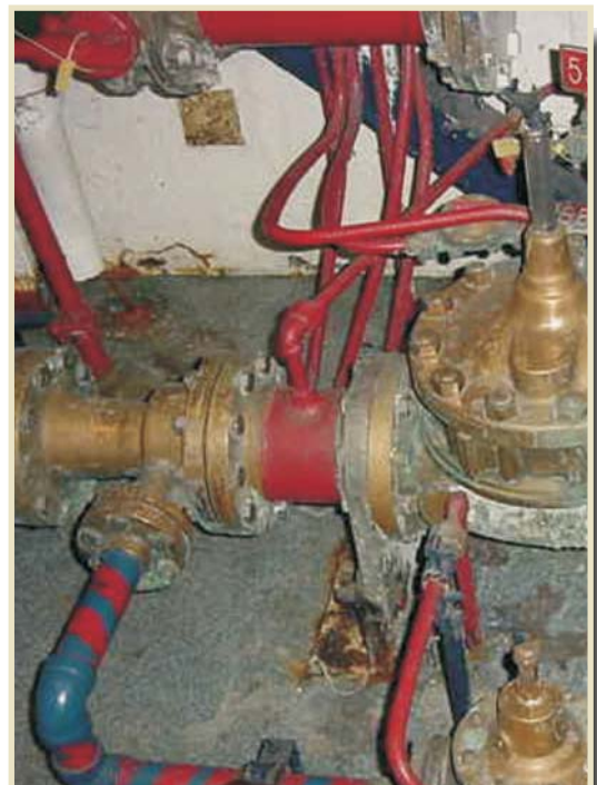
AFFF Station 5 Years ago.
