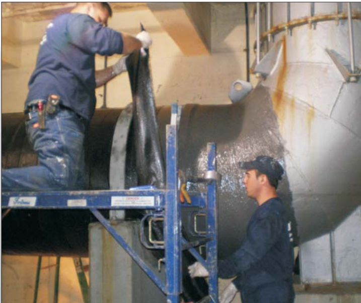
DuraWrap Carbon Fiber, impregnated with DuraWrap Polymers, being wrapped around pipe section.
