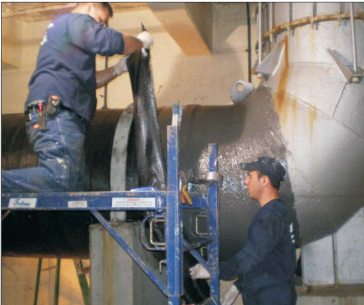
DuraWrap Carbon Fiber, impregnated with DuraWrap Polymers, being wrapped around pipe section.
