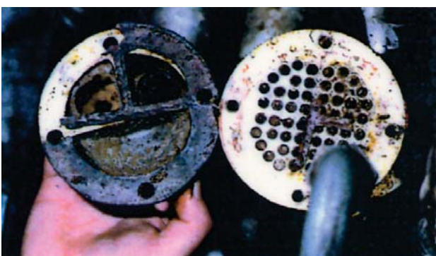
Mineral scale on T.C.U. completely eliminated in just one month.
