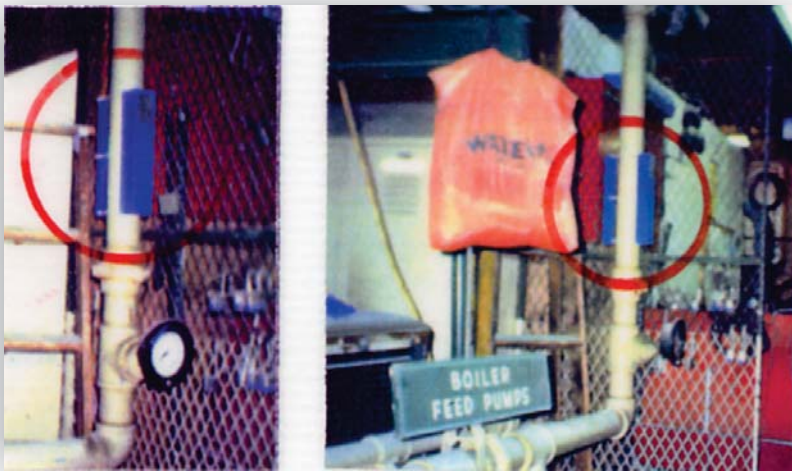
ENEFLOW 5000's installed on boiler feed line.
