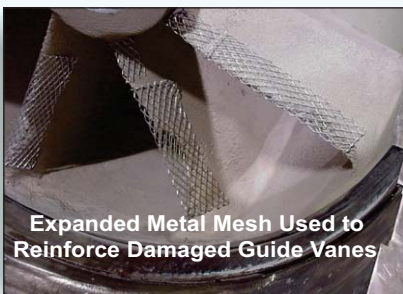
Damaged Guide Vanes
