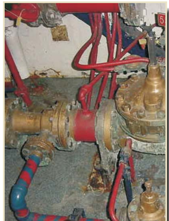
AFFF Station 5 Years ago.
