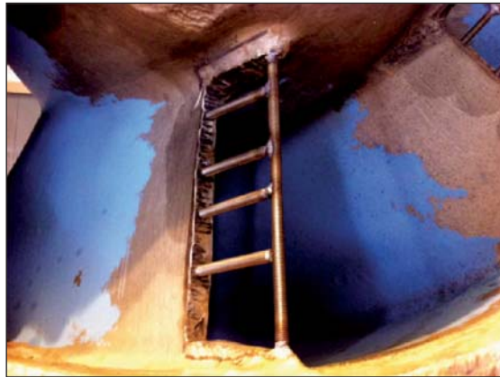
A threaded rod "skeleton" was installed by tack welding to the already cut vanes.
